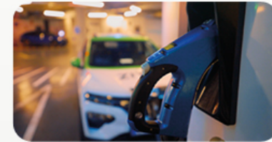
EV chargers at the hub "Canalejas 360"
