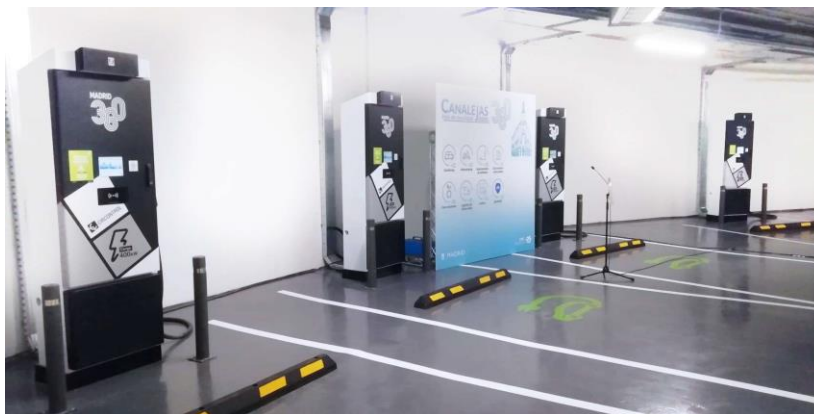
Figure 16 EV chargers at the hub "Canalejas 360"
